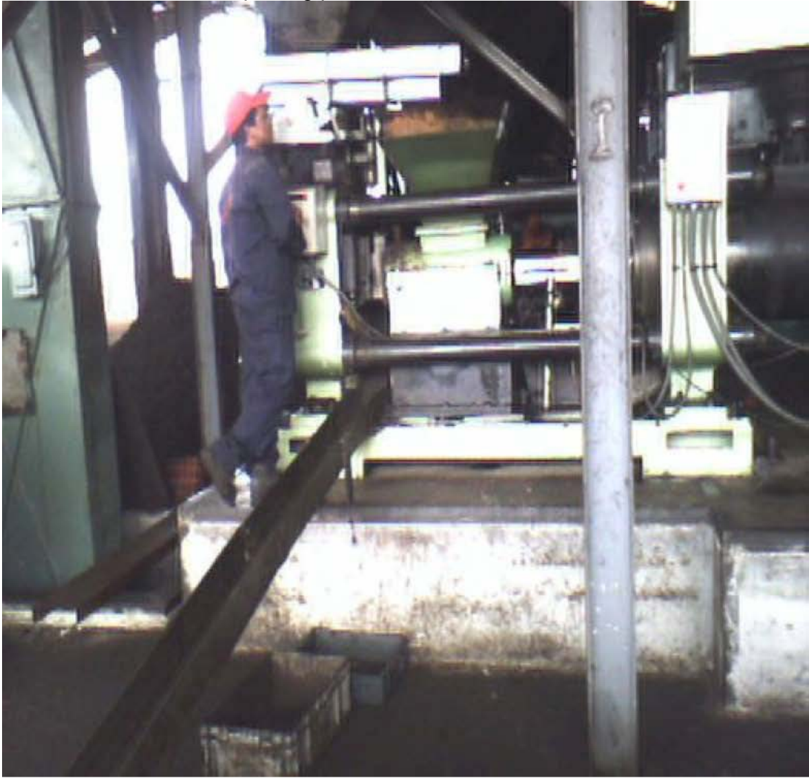
Briquetting press used in Mexico – Steel
